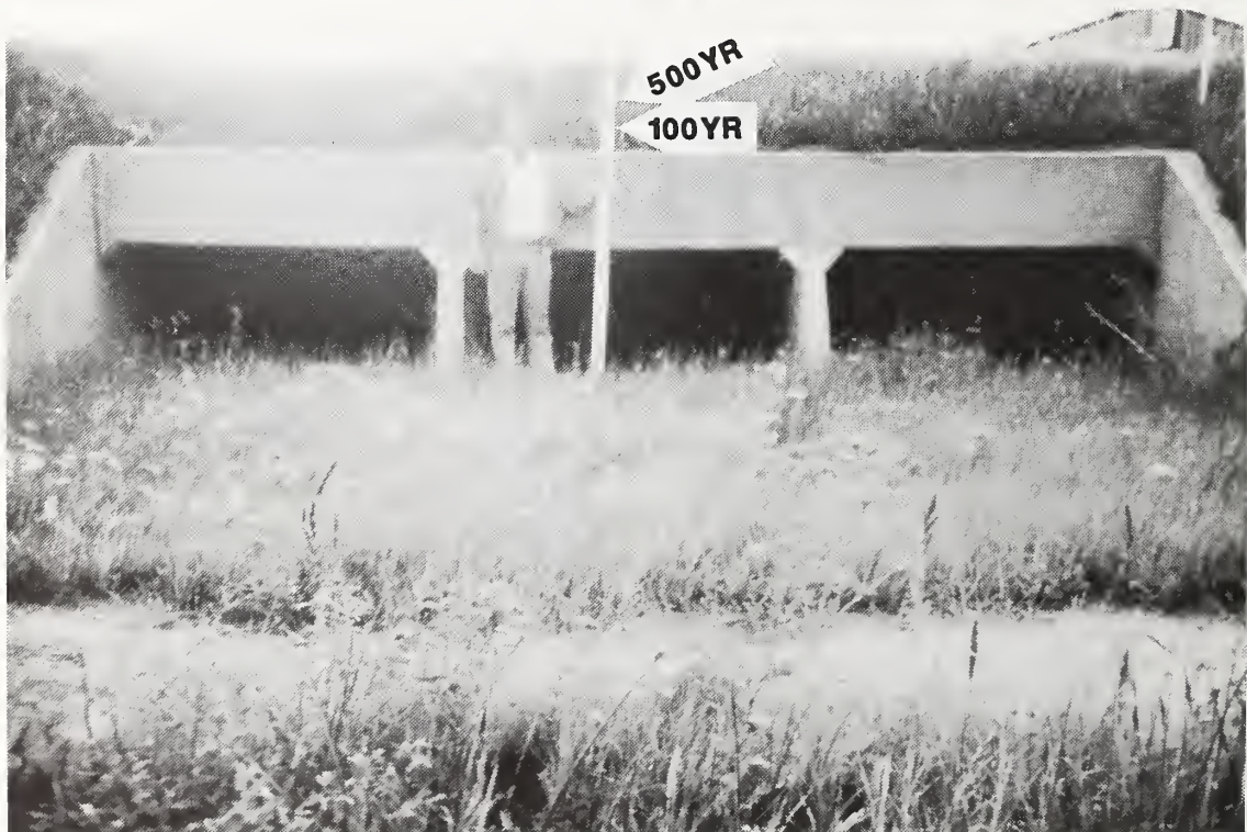
MILE 2.08 - HIGHWAY 2 AND 85 SW ¼ SEC.12, SE ¼ SEC.11, T154N, R101W Looking Downstream
